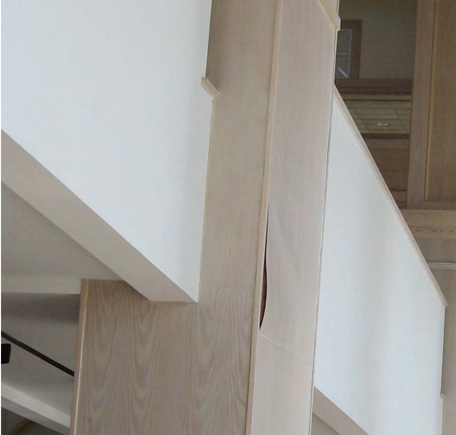
Millwork Water Damage Precedent to Hurricane
