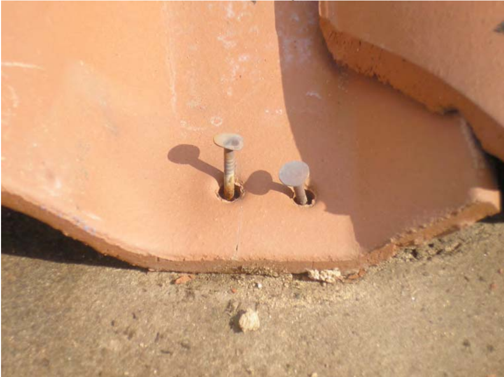
Roof Tile Attached With Non-specification Fasteners
